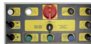
• Quadro comando • Control panel
